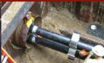
Ronkonkoma Hub Pump Station
