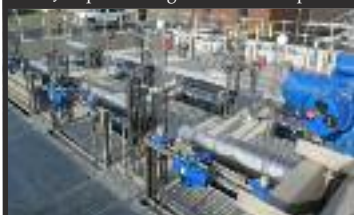
Bergen Point WWTP
