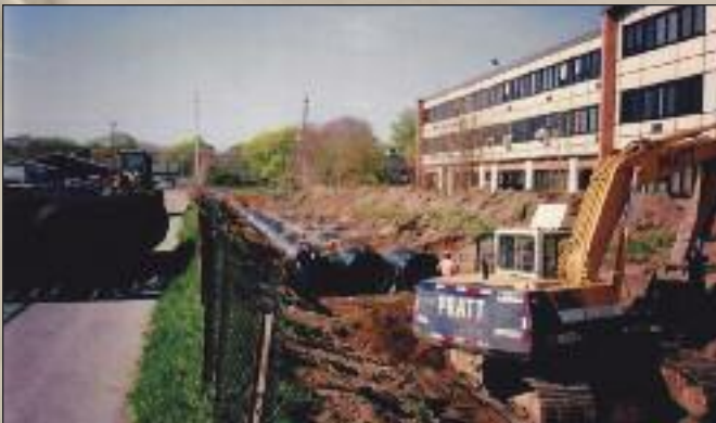
Photos (Courtesy NC DPW) Above: LICA member Pratt Brothers at work on Nassau Co. sump and drainage maintenance project at MacArthur HS (1996). Opposite page, top: Making progress on the new Nassau Co. Police Academy.
